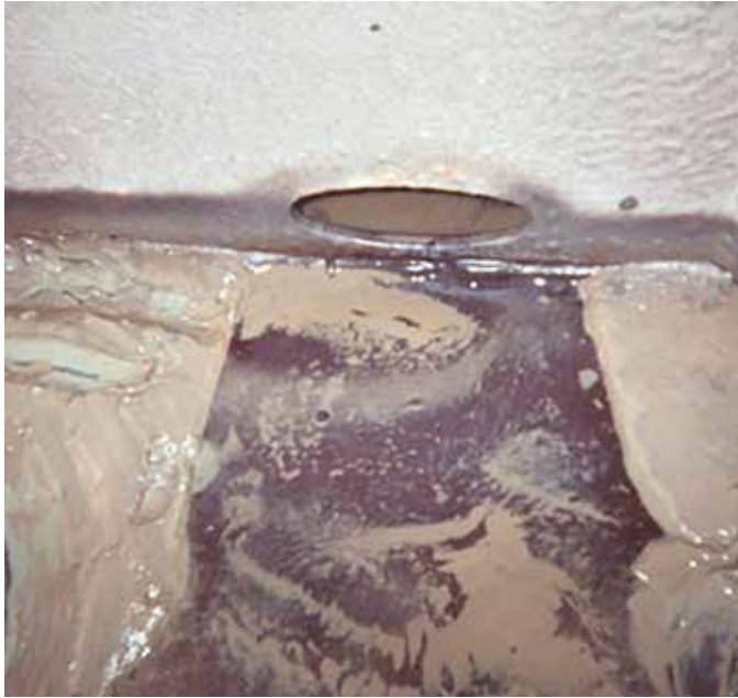
Figure 2: Sediments accumulate in ballast water tanks in areas with flow stagnation.
