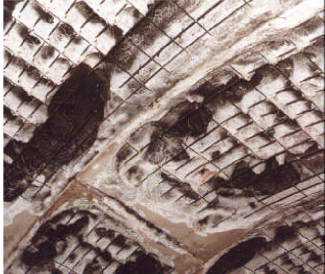
Figure 14: Channel Tunnel fire damage
