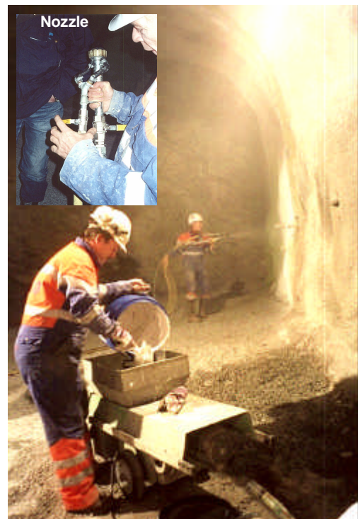
Figure 12: Using a simple screw pump, two men can apply sprayable membrane up to 50m 2 per hour
