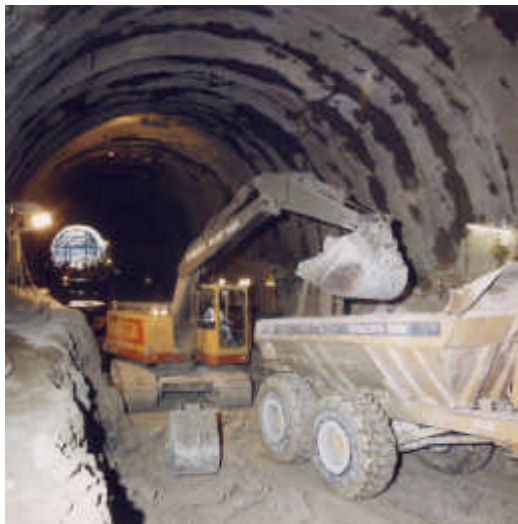
Figure 10: Water ingress through sprayed concrete containing steel reinforcement
