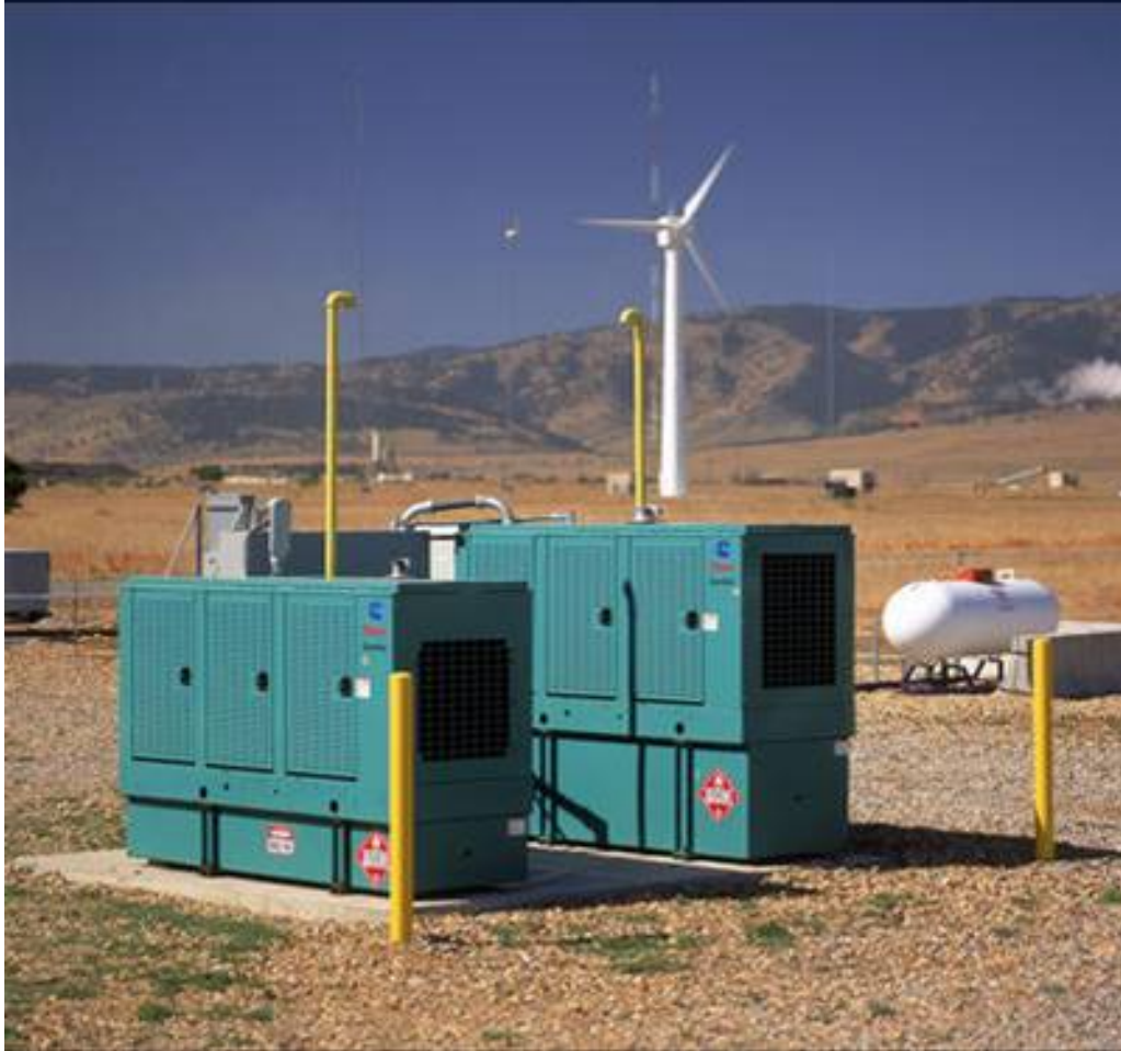
Figure 38. Internal combustion engine-generator systems (NREL 2008)
