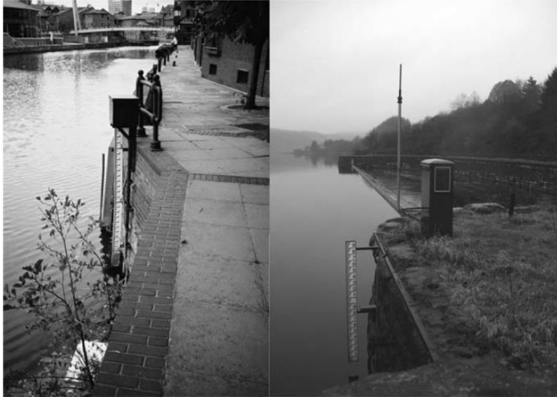
Examples of pressure transducer installations with associated gauge boards (a) river level gauge (b) reservoir gauge (Sene 2008)
