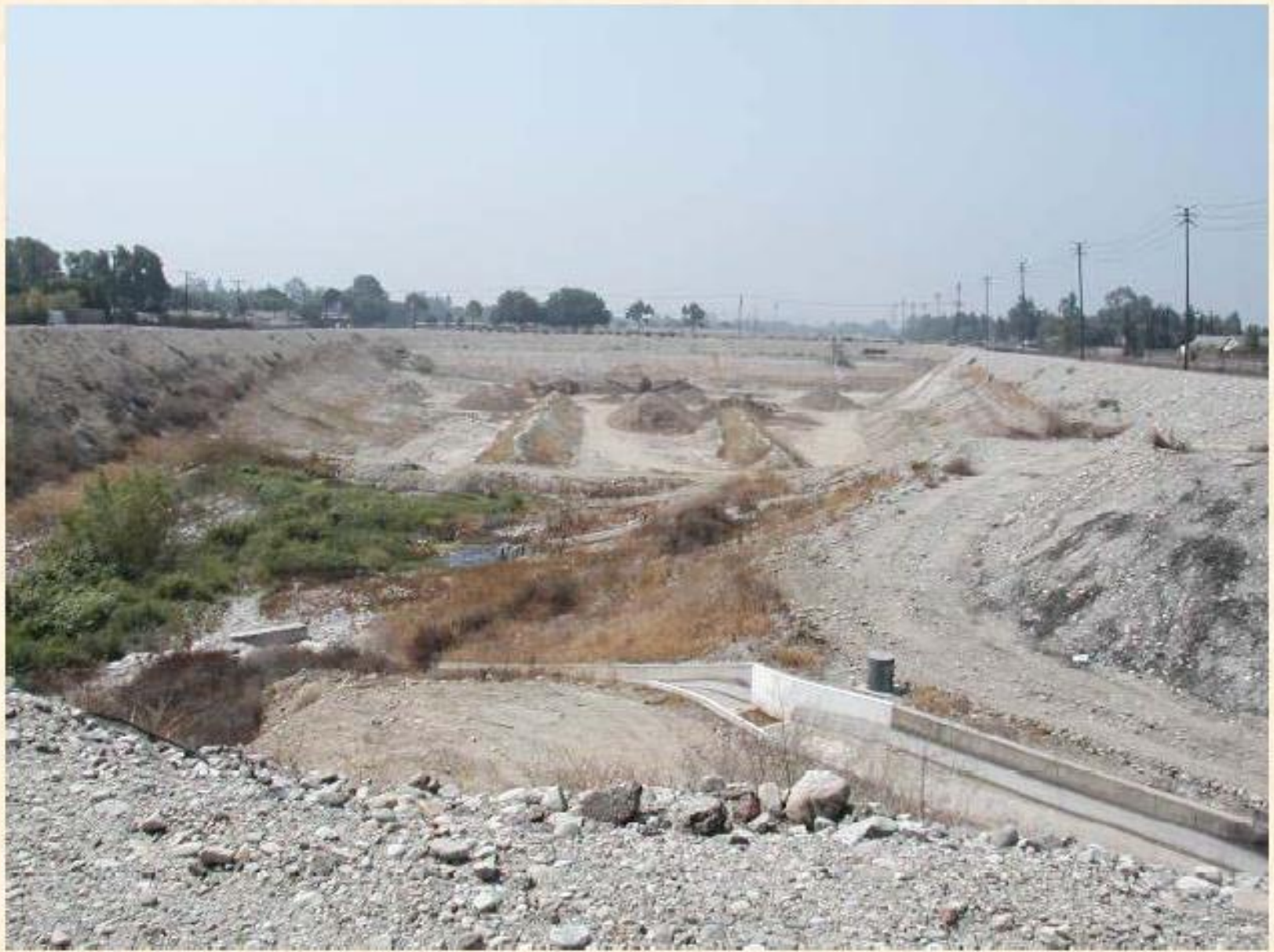
Montclair Basin No. 2 looking south with storm water inlet in foreground (Owner: CBWCD)
