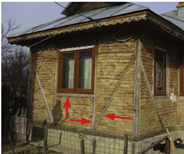
Fig. 17. Structural timber elements in “paianta” houses: columns and braces which do intersect at the bottom.
