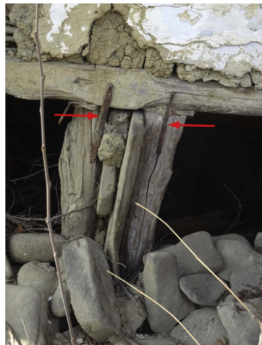
Fig. 22. Detail of pile foundation connected to the bottom beam with steel clamps.
