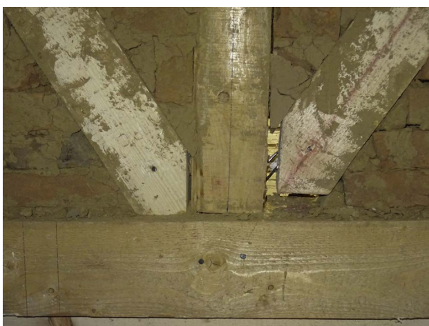
Fig. 39. Bottom middle connection with significant pull-out of one diagonal brace.
