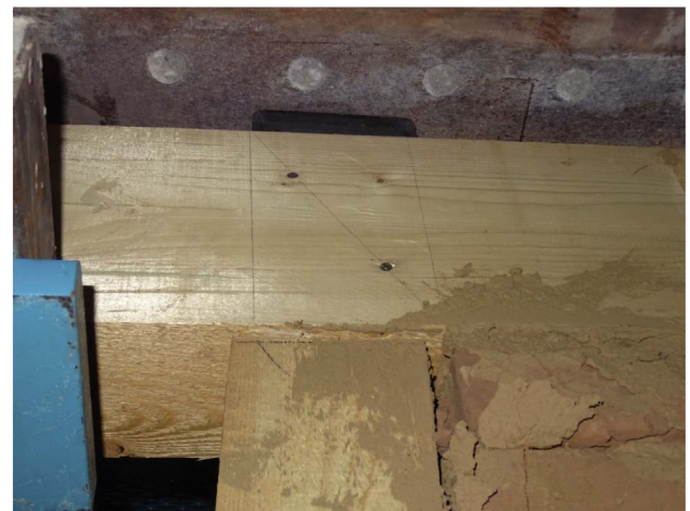
Fig. 40. Upper marginal connection with imperfect executed connection (initial defect).
