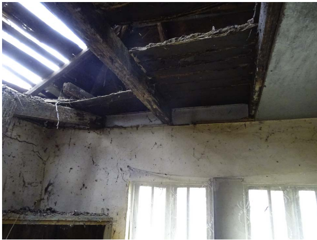
Fig. 23. Detail of floor in an abandoned house.
