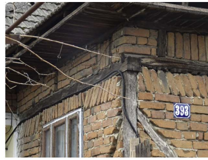
b. The diagonals are stopped below the upper connection between beam and column, and the last row of bricks is laid in an inclined position
