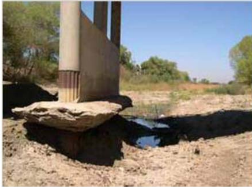
Figure 2.17 - Scouring around a bridge foundation
