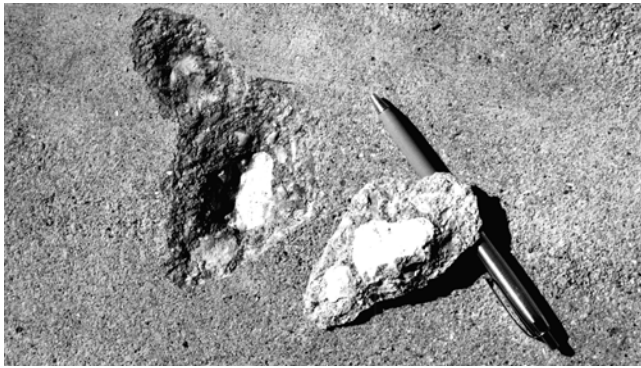
Fig. 6—Pop-out due to unsound aggregate particle.
