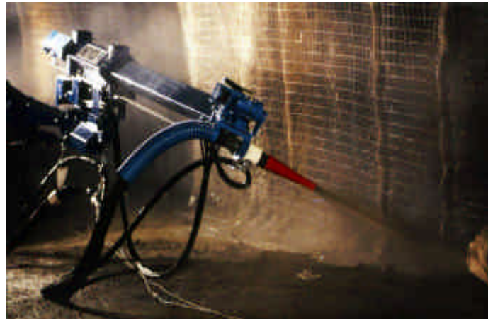
Figure 4: Robotic manipulator for safe, high output and quality wet-mix sprayed concrete application
