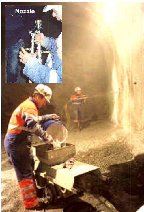
Figure 22: Using a simple screw pump, two men can apply sprayable membrane up to 50m 2 per hour
