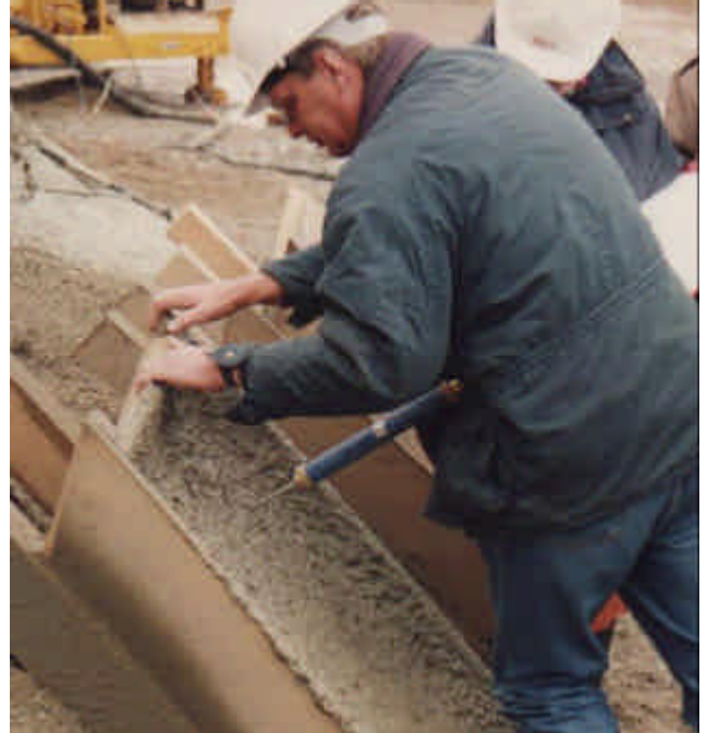
Figure 25: Traditional Proctor penetrometer where full body weight required (Jubilee Line Project, UK, 1994)
