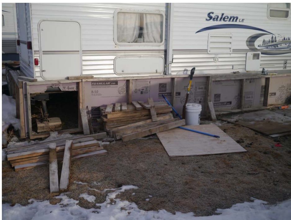
FIGURE 4. Installing insulation in preparation for the North Dakota winter in the Bakken oil patch (W. Caraher).
