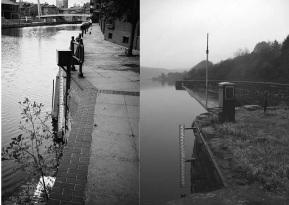
Examples of pressure transducer installations with associated gauge boards (a) river level gauge (b) reservoir gauge (Sene 2008)
